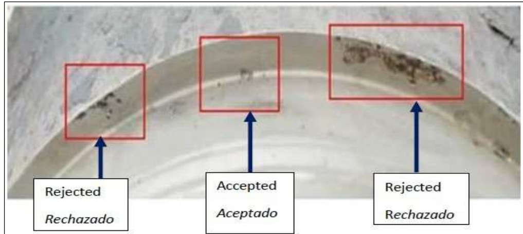
Photo.21 Pitting on external shoulder of a FMAX pin connection.
