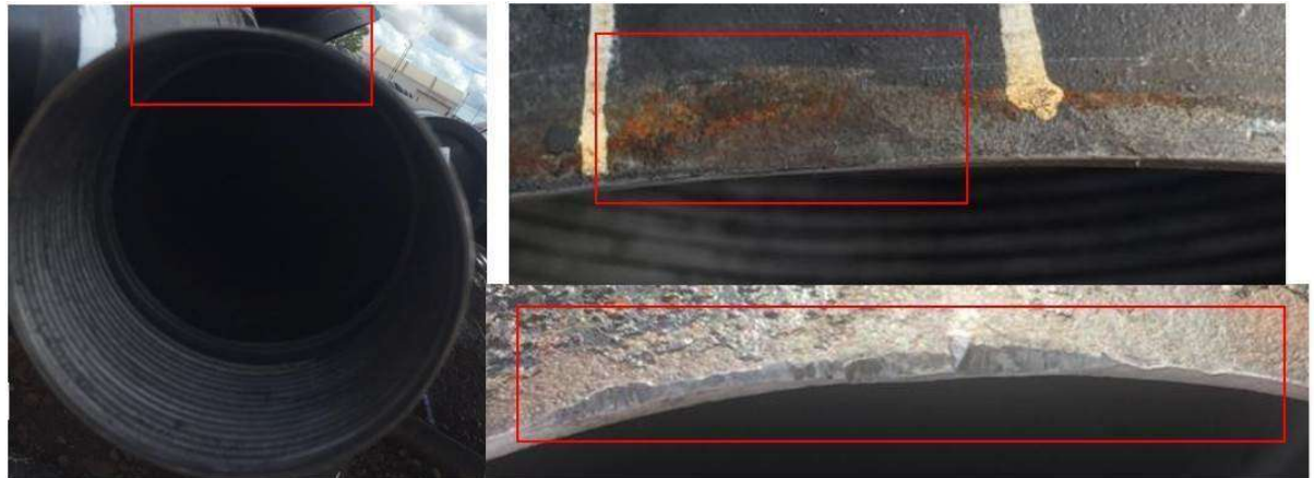
Photo.19 FMAX Box, the connection was damaged during transportation: Rejected
