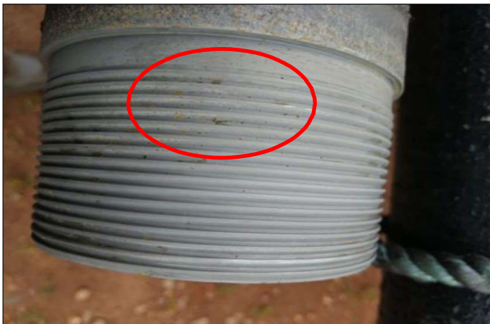
Photo.15 Minor Oxidation: Can be repaired
